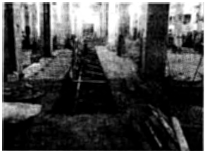
One of the communications trenches in the basement.
