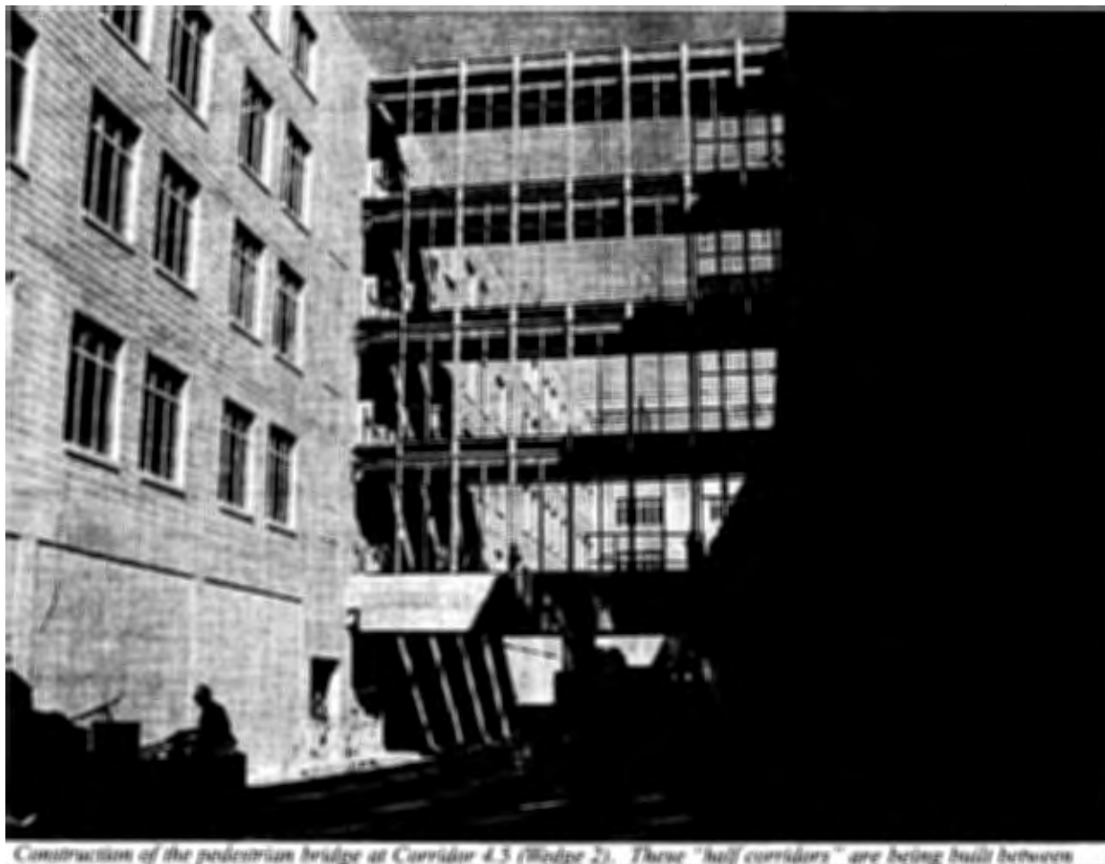
Construction of the pedestrian bridge at Corridor 4.5 (Wedge 2). These "half corridors" are being built between all ten of the Pentagon's radial corridors to increase accessibility and building circulation.
