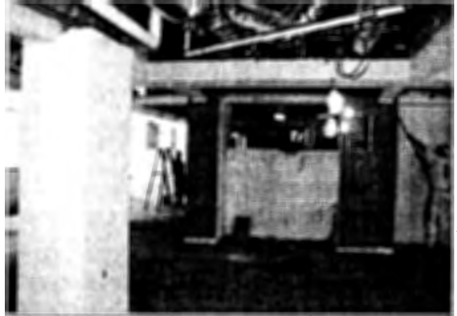
Workers finishing the drywall in a Wedge 2 space. Much of the Tenant fit-out work has been completed.
