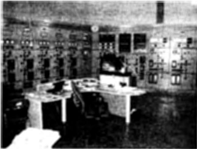
The control room for the RDF's Emergency Power Facility.
