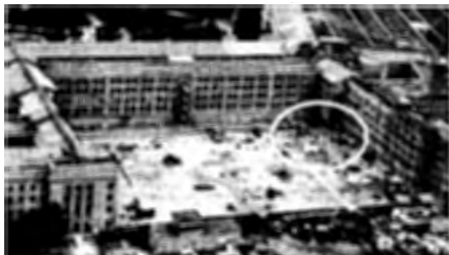
November 27 - After one month and one day, crews completed the demolition phase of the Phoenix Project. This photo shows the initial column formwork (circled) to support the 2nd floor.
