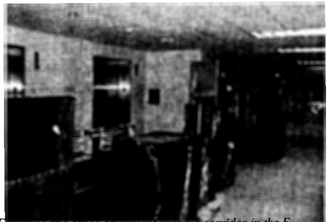
Furniture and office equipment lining a corridor in the E-Ring, ready to be placed into renovated office spaces. These were the first Phoenix Project offices to be reoccupied.
