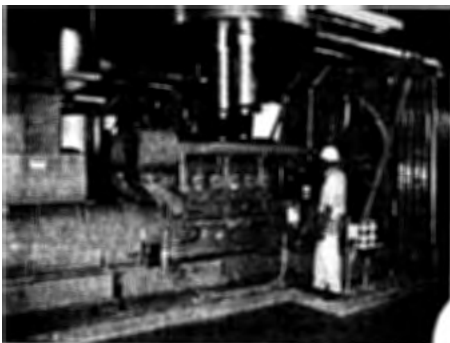
One of the RDF's emergency power generators
