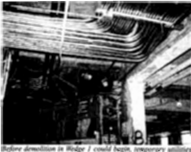
Before demolition in Wedge 1 could begin, temporary utilities and communication lines had to be installed.
