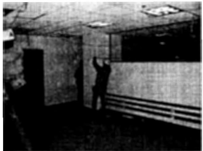
Workers installing the "smart walls" and other tenant fit-out work in Wedge 2.
