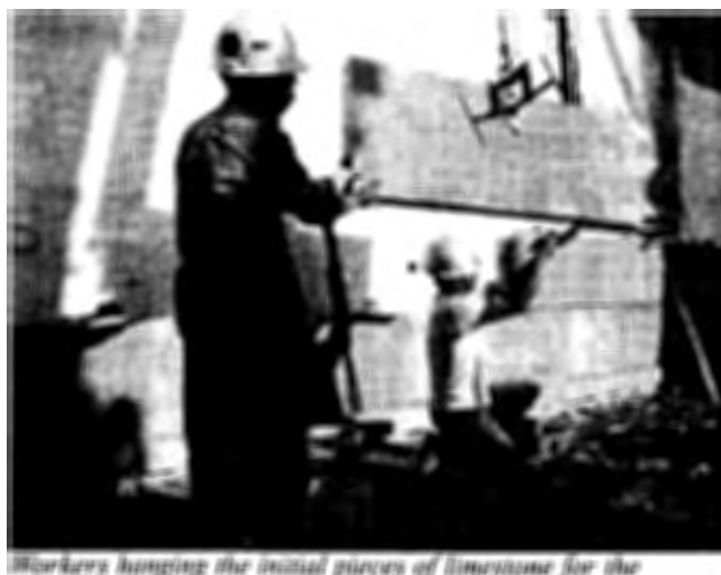
Workers hanging the initial pieces of limestone for the building facade. The building's new and original limestone came from the same vein in Indiana.
