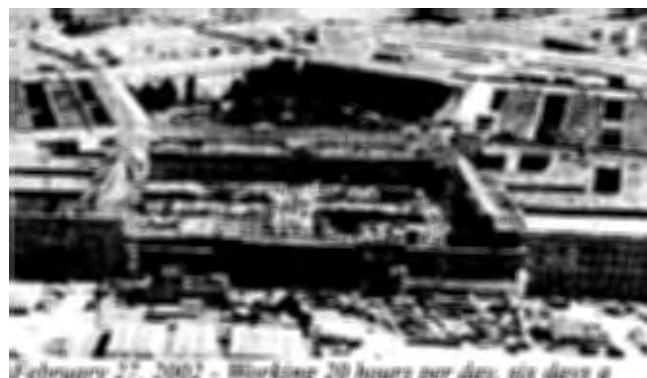
February 27, 2002 - Working 20 hours per day, six days a week, construction crews made tremendous progress on the Phoenix Project structure.
