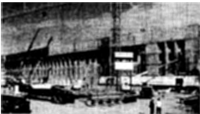
On April 5, construction crews made the final concrete pour, finishing the Phoenix Project structure.
