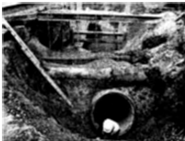
Workers install outfall pipe below an existing telephone ductbank and water line at a local roadway.
