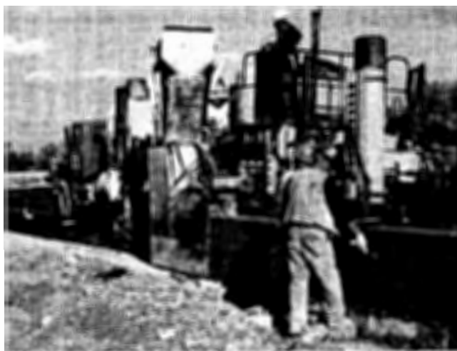
Workers using a slip form machine create the median barrier for the southern tie-in of Highway 110.
