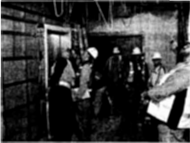
Inspection of a Wedge 2 elevator.
