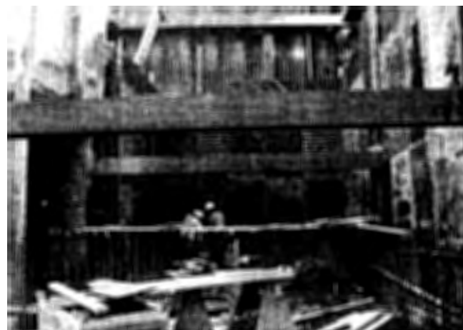
Workers install wall forms at the screen house. First level was placed on Nov. 14, 2003.
