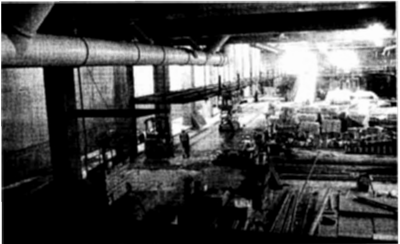
Internal view of the PAC under construction. Visible to the left is the construction of the suspended running track.
