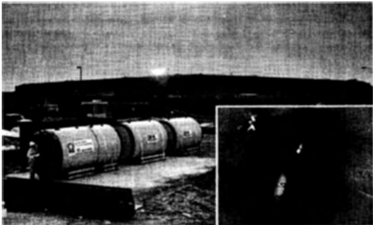
A look at pieces of the micro-tunneling machine that places the underground pipe system for the Intake/Outfall project.
