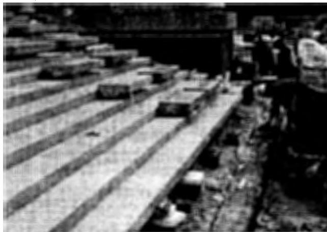
Crews working to replace the steps at the Mall Terrace entrance. The stairs needed to be partially demolished during waterproofing of the parking lot.
