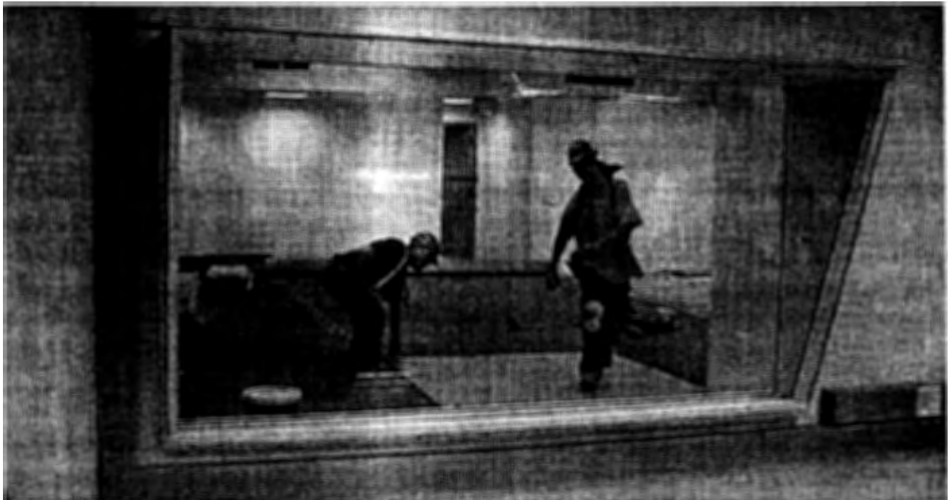
This photo shows workers installing carpet in the new OSD Press Briefing Room. The picture was taken from the audio visual control room next door.
