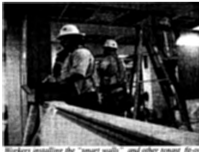
Workers installing the "smart walls" and other tenant fit-out work in Wedge 2.
