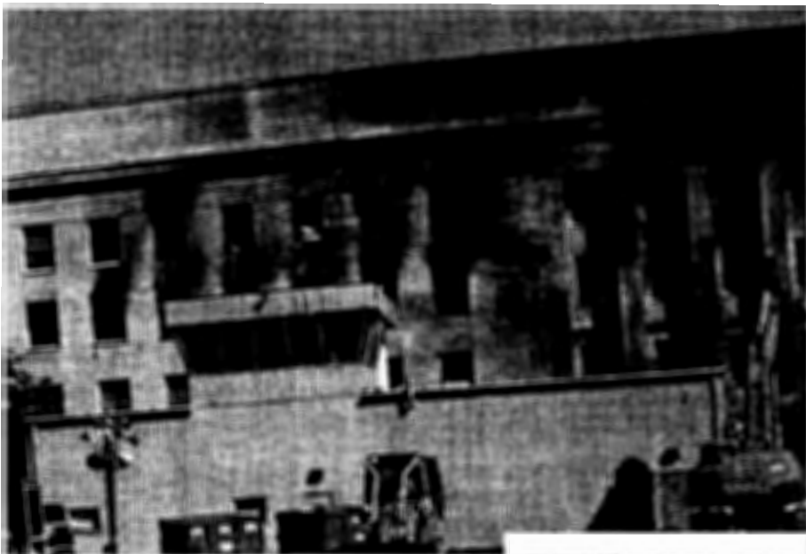
Left: The demolition of the heliport tower damaged in the September 11 attack was one of many smaller projects undertaken by the Ancillary Team.
