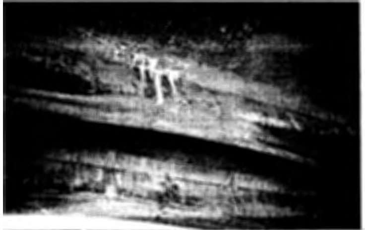
Deteriorated River Terrace Vehicle Bridge
