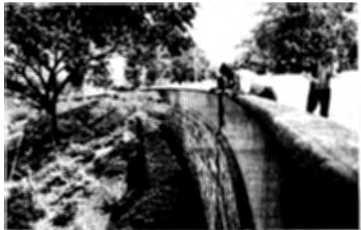
Deterioration at wall on North Parking Pedestrian Ramp
