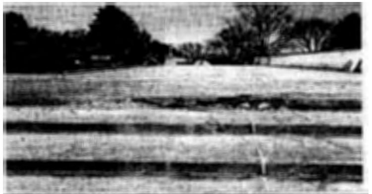
Typical Deterioration of River Terrace
