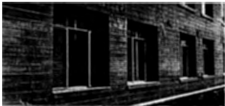
Typical Exterior Walls Needing Repair
