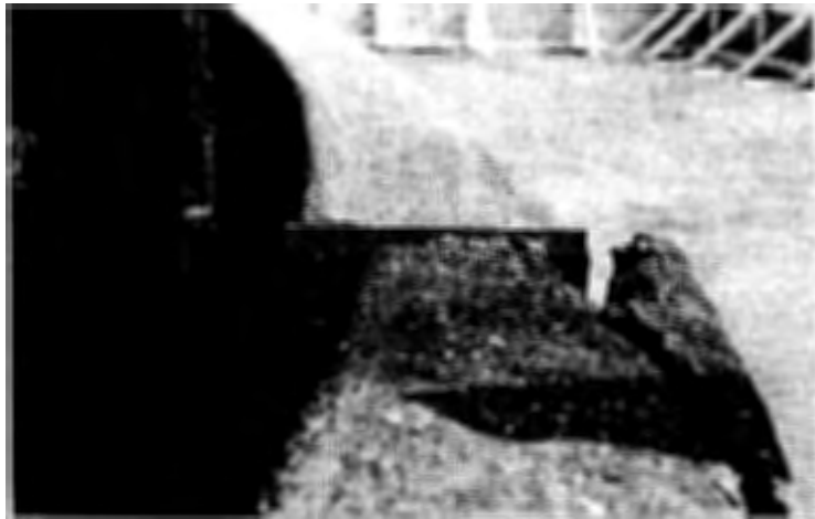
Deterioration at North Parking Pedestrian Ramp (Close-up of wall)
