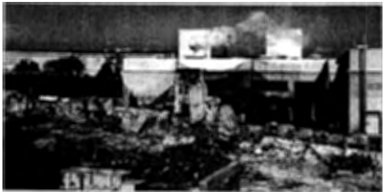
Old Heating & Refrigeration Plant Virtually Demolished with New Heating & Refrigeration Plant in the Background
