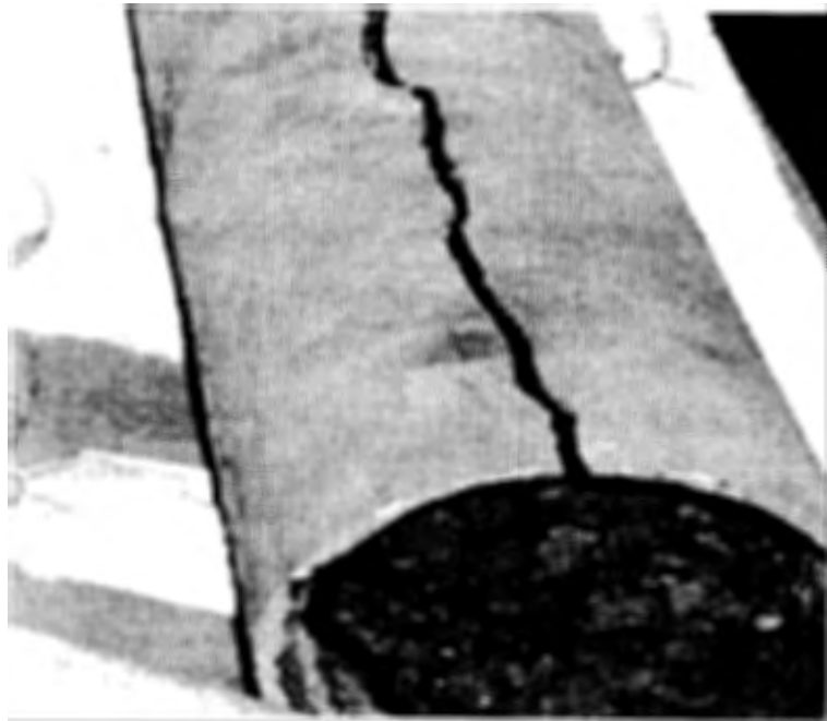
Vertical Sanitary Riser Pipe Split from First to Fourth Floor
