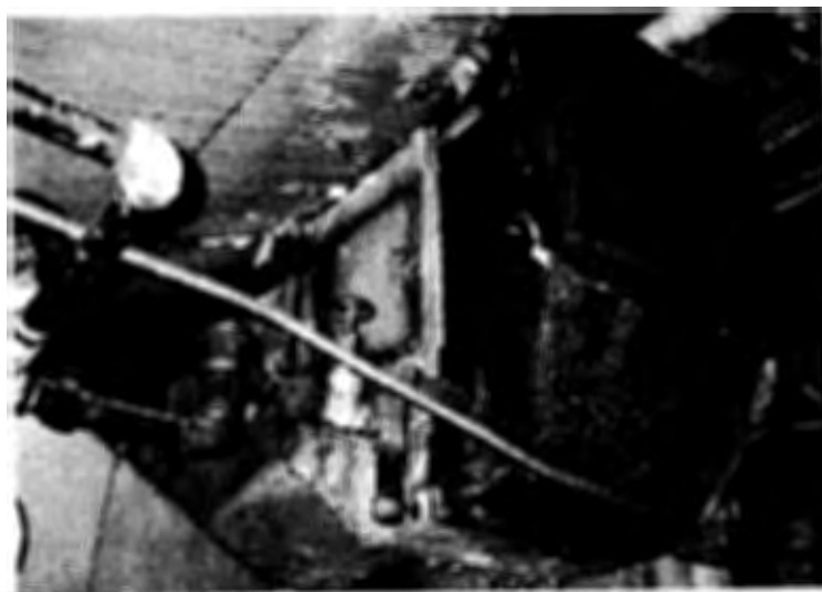
Typical Ductwork Surrounded by Asbestos Insulation
