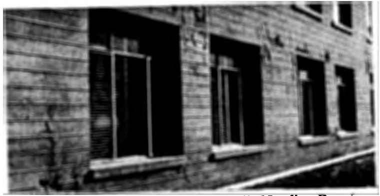
Typical Exterior Walls in Light Wells Needing Repair
