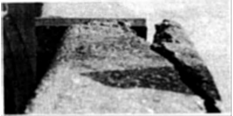
Deterioration at North Parking Pedestrian Ramp Leading to the Corridor 8 Entrance.
