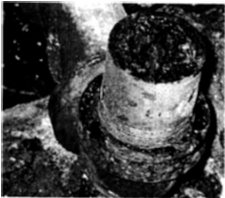
Typical Example of Drain Pipe, Clogged After Years of Deposits and Deterioration.
