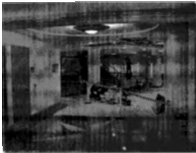
In Wedge 3, the escalators at the apex of Corridor 7 & 8 are nearing completion.
