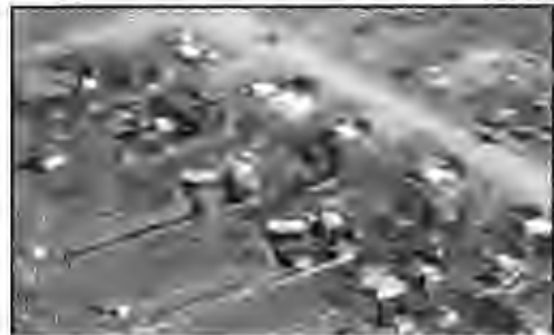
Figure 7: Missile Field 2 at Fort Greely, Alaska under construction in September 2009. Construction of the 14 silo field will be complete in FY 2012.
